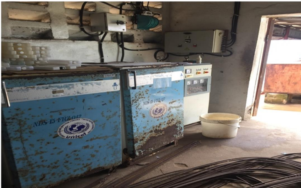
Photo 1: Construction materials in the National Vaccine Store which also housed refrigerators (seen) for Montserrado county depot.
