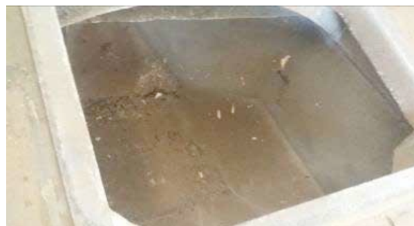
Non-functional incinerator at General Hospital Gwadabawa, Sokoto State
