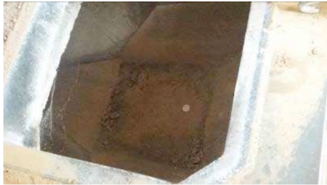
Non-functional incinerator with Cobwebs inside at Wamako Orthopaedic Hospital in Sokoto State
